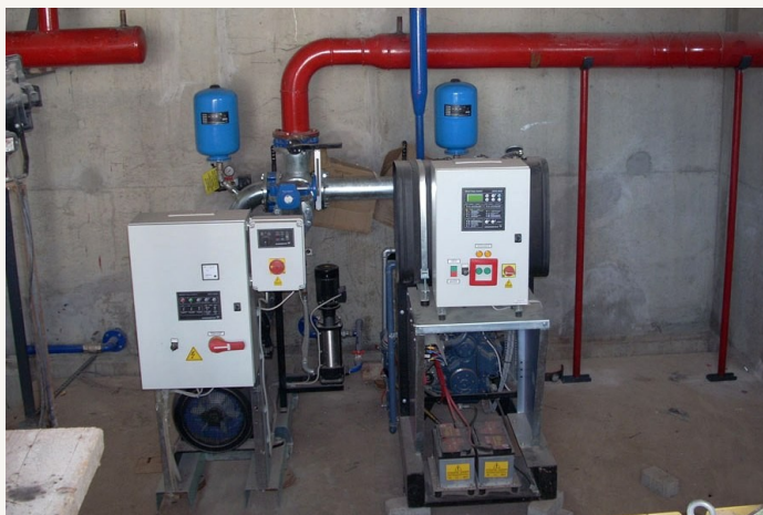
Fire-protection technical system: pumps and distribution.
