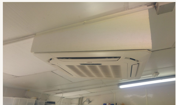
Cassette air conditioning • Madrid workshop.
