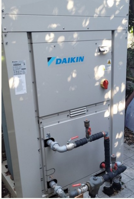
Daikin chiller / chilled-water generation.
