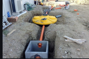
Water treatment / purification.
