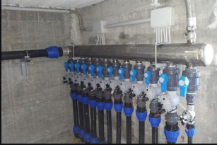
Water distribution and manifolds.
