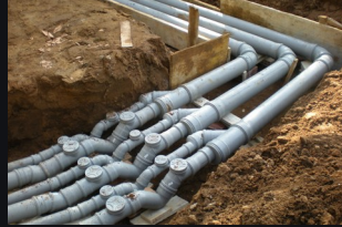
Underground networks and drainage.
