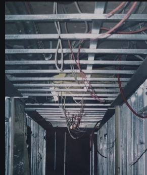
Distribution routes and systems above the corridors.
