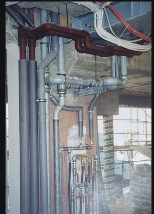
Risers and technical networks.
