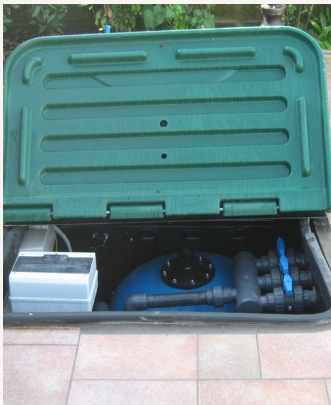
Underground plant room.
