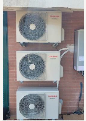
Outdoor units / distribution.
